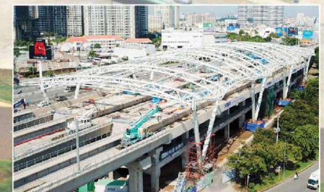
Metro Station Sai Gon - Suoi Tien Line 1
